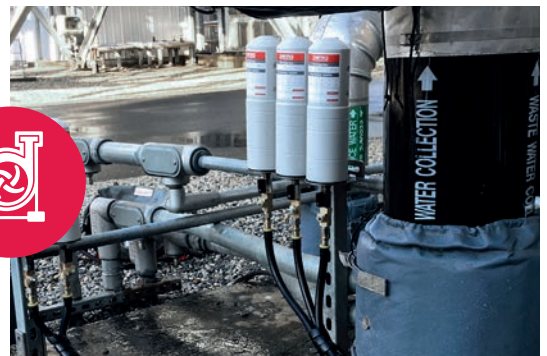
Industry: Power Generation Application: Pumps
